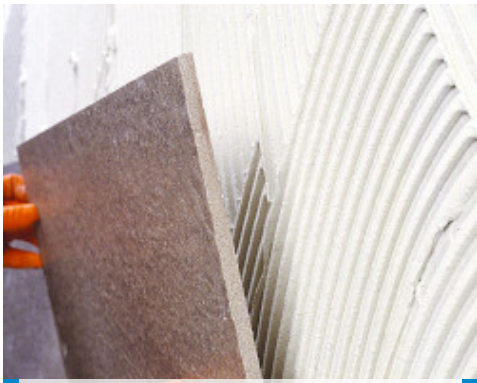
Laying large-sized, double-fired tiles on wall starting at the top and working downwards
